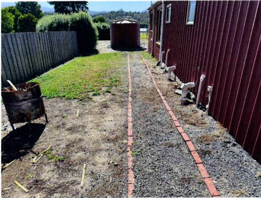
Plate 2 – Wastewater fixtures exiting the building on the northern side - looking to the east.
