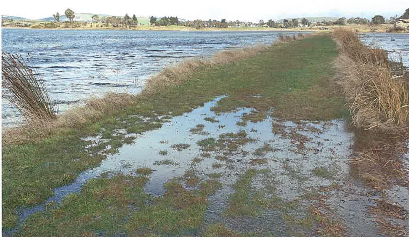
Section of the large bund wall where the water is flowing over to the rear of the lake. 2 nd Sept 2024.
